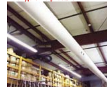
Shown is the M/FA fabric duct installed at State Automatic Heating & Cooling.
